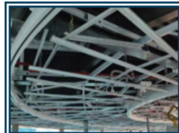
Under Ceiling Monorail Track
